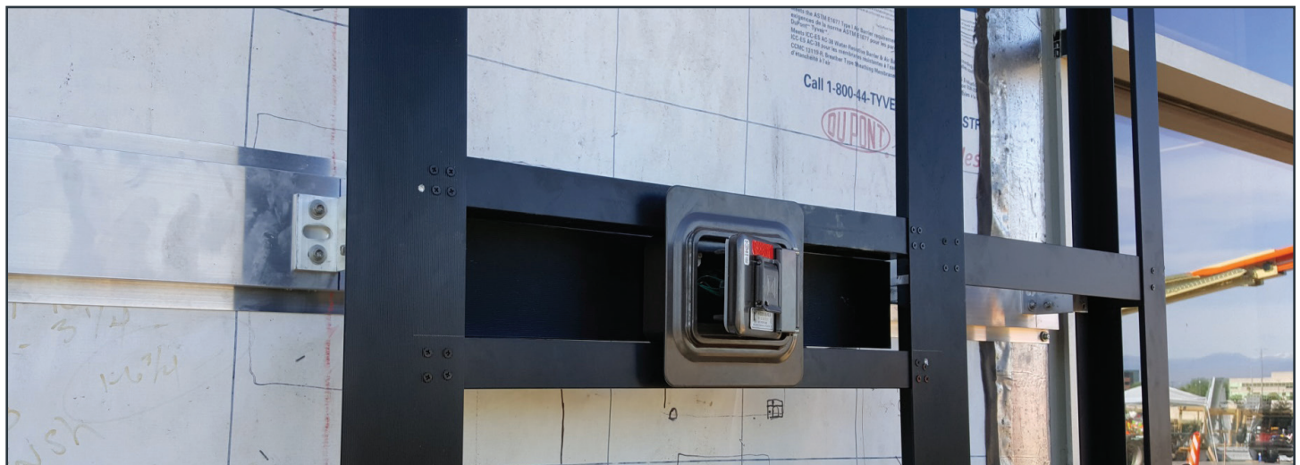
Example of box for firefighters installed on and with our system.
